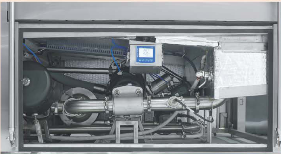
Figure 2 | Sloped piping in a pharmaceutical-grade washer
