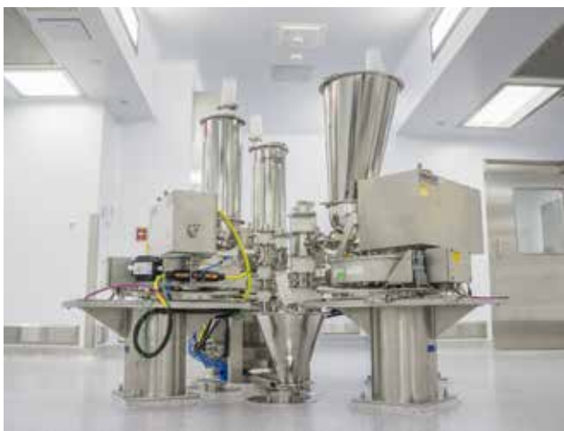
Second floor feeders, Puerto Rico
