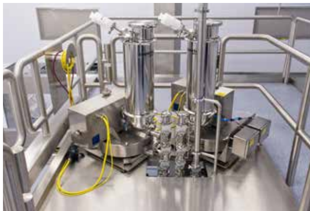
API feeders on vibration isolation pad, Indianapolis
